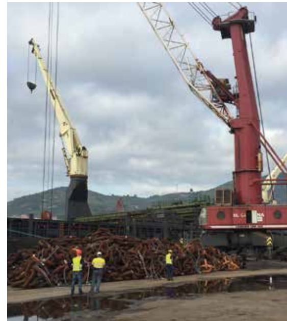
Chains being carefully loaded onboard the vessel by means of 2 port cranes who worked simultaneously.
